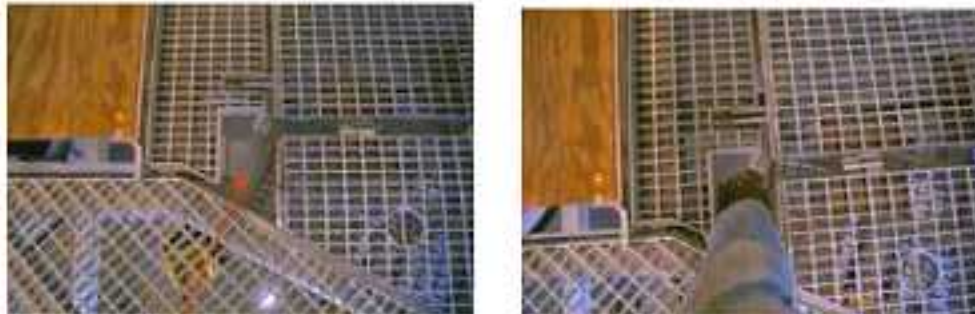
Void in L3 floor
