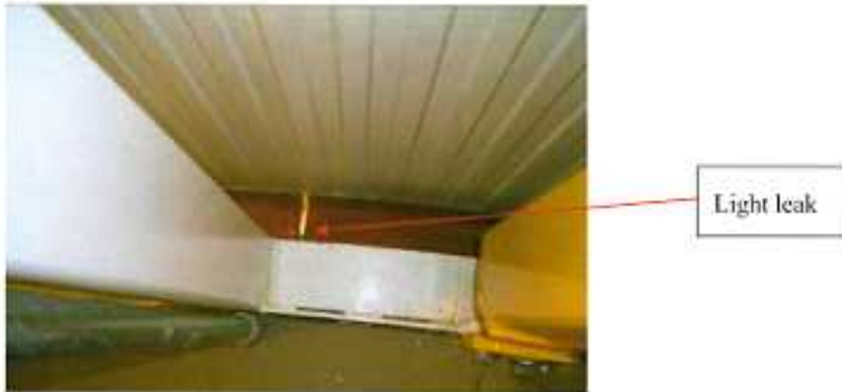
Figure 21 Ring Wall seal light leak
