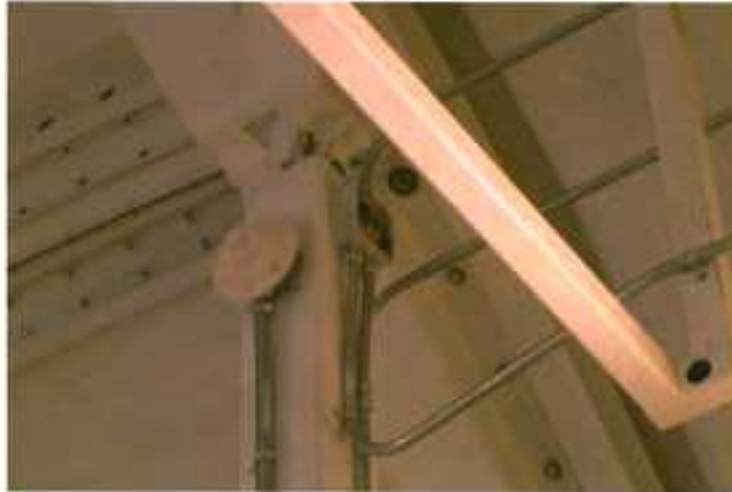
Figure 20 THUD box on Hanger
