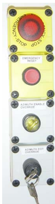
Lick Emergency Controls: ESTOP, E-RESET, Azimuth Override, End Of Travel Override
