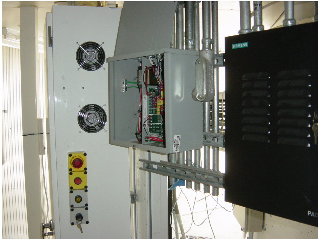
Lick Emergency Response Controls On Drive Cabinet
