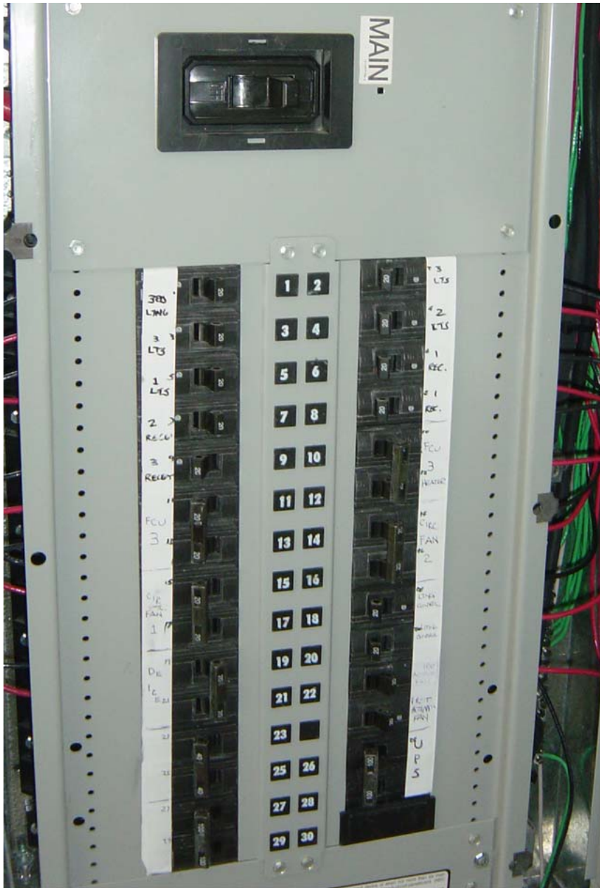
Lick Power Distribution Switchboard
