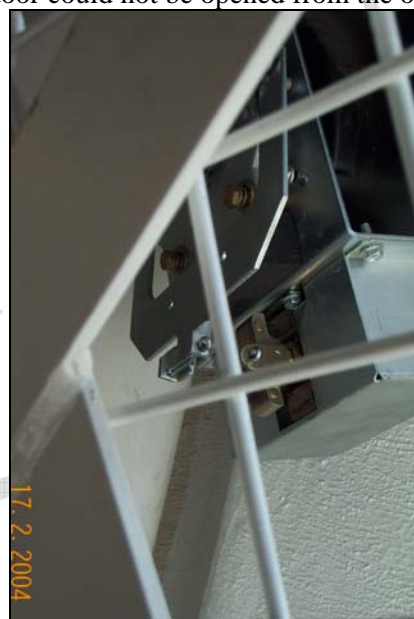
Brake Prior To Removal
