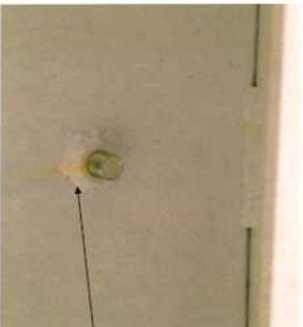
Slight staining around skirt attachment screw, inside Azimuth beam
